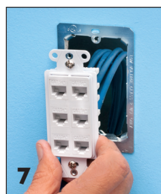
7 Wire low voltage device.
